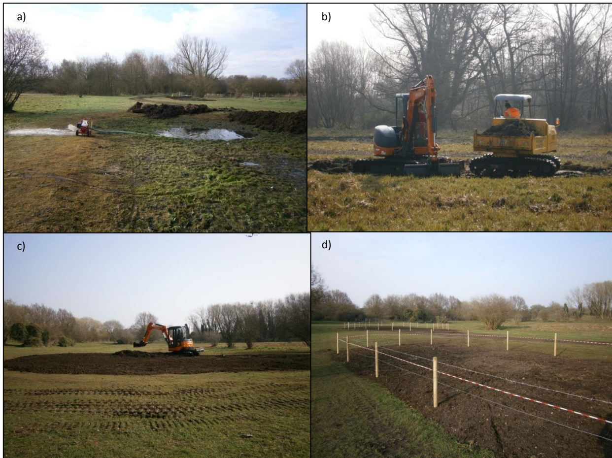
Figure 2. Operations to control C. helmsii : a) Draining and filling existing ponds, b) excavating new ponds, c) levelling excavated material, d) fence posts, wire and tape erected.
