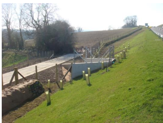
Figure 2. Culvert 10, showing line of trees (known horseshoe bat flight-line) leading towards southern entrance, marked by white wing-walls. Tree guards indicate the planting around back and sides of the culvert to guide bats into the structure.
