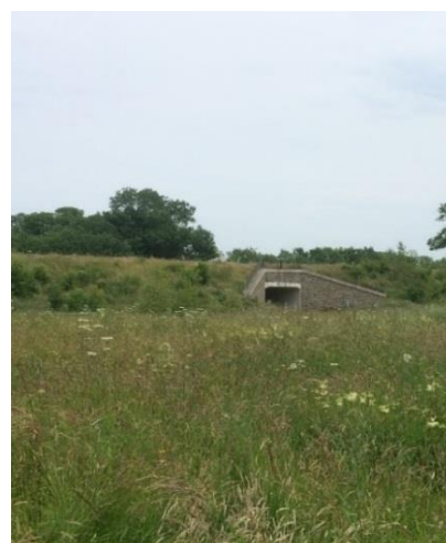
Figure 5. Southern entrance to Sunnyside Underpass (for cattle), located within a retaining wall created within the road embankment to avoid loss of habitat from Sunnyside Wood.
