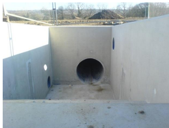
Figure 3. Culvert 5, a 1.5 m diameter drainage ring (with steps leading down into the entrance for otters).
