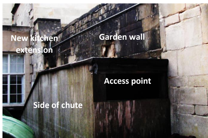
Figure 5. Current chute in place (after several years).
