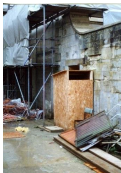
Figure 3. Initial chute design (implemented in 2000). The photograph shows a temporary chute (initial design), the doorway (just visible behind chute) leading to the steps down into the basement, and the courtyard (garden) wall. The boiler house is behind the photographer (photo taken prior to work on the new kitchen extension).
