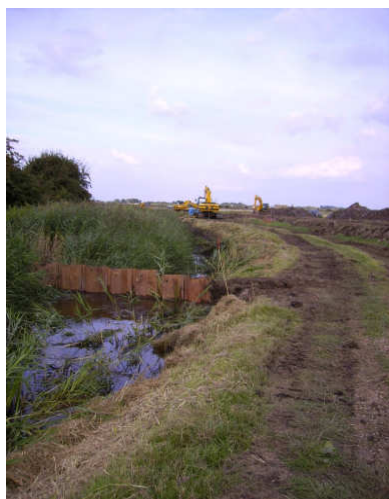
Figure 4. Steel piling used to subdivide existing soke dyke habitat as works commenced to infill dyke, August 2006.
