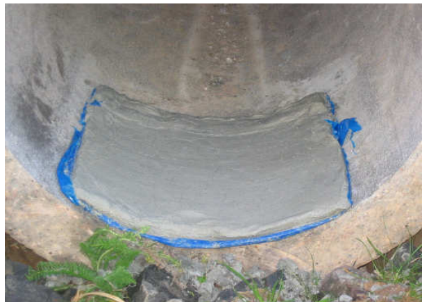
Figure 1. Installation of a clay drain seal at the entrance to a dry culvert (Photo: Dorian Latham)
