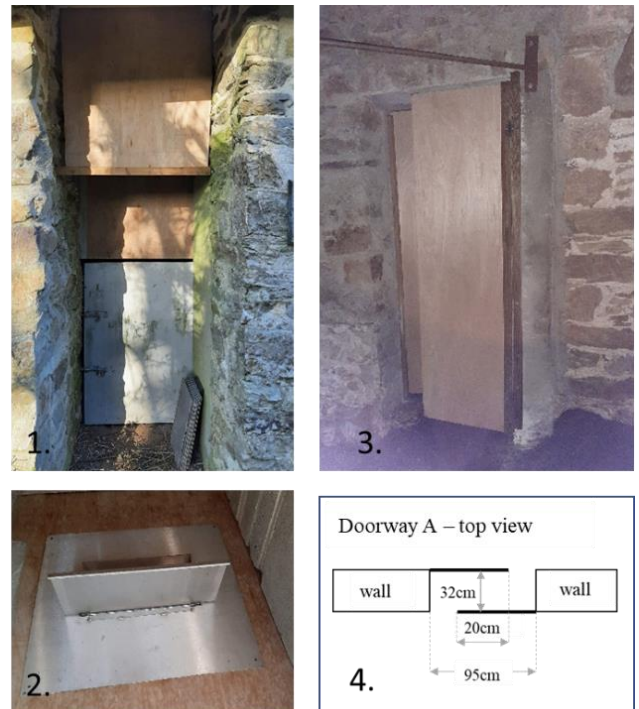
Figure 2: Entrance A with light baffle (1) and tip tray (2). The tip tray is a tilting tray made of 3mm thick aluminium, attached with hinges to a vertical metal sheet that forms a frame around the opening where the tray sits. The vertical metal surface (666 mm x 538 mm) and tray (390 mm x 170 mm) are smooth and prevented owls or other predators gripping the surface. Doorway A with baffles (3) and dimensions (4). Two wooden baffles were fitted on each doorway, attached to opposite sites and parallel between them, mounted on hinges to allow for human access.
