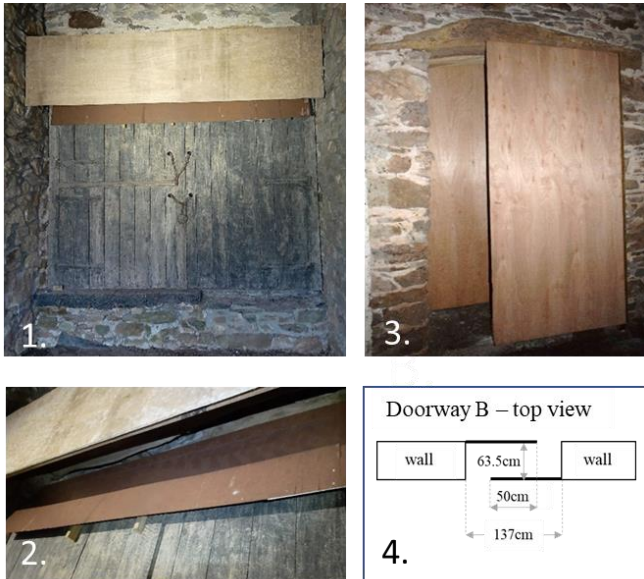
Figure 3: Entrance B (1) with baffle and metal tray (2) fitted as an anti-gripping surface to prevent owls perching. Doorway B with baffles (3) and dimensions (4).
